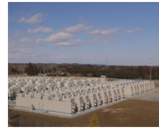
Stationary Battery Energy Storage Systems
