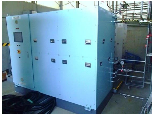
2015 Hydrogen station in Kyushu Univ. (1Nm 3 /h)
