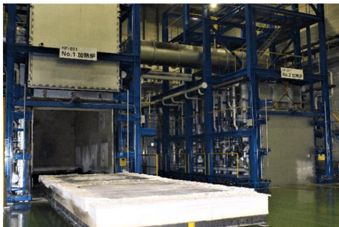
The furnaces to inactivate batteries of ECO-SYSTEM AKITA CO., LTD.
