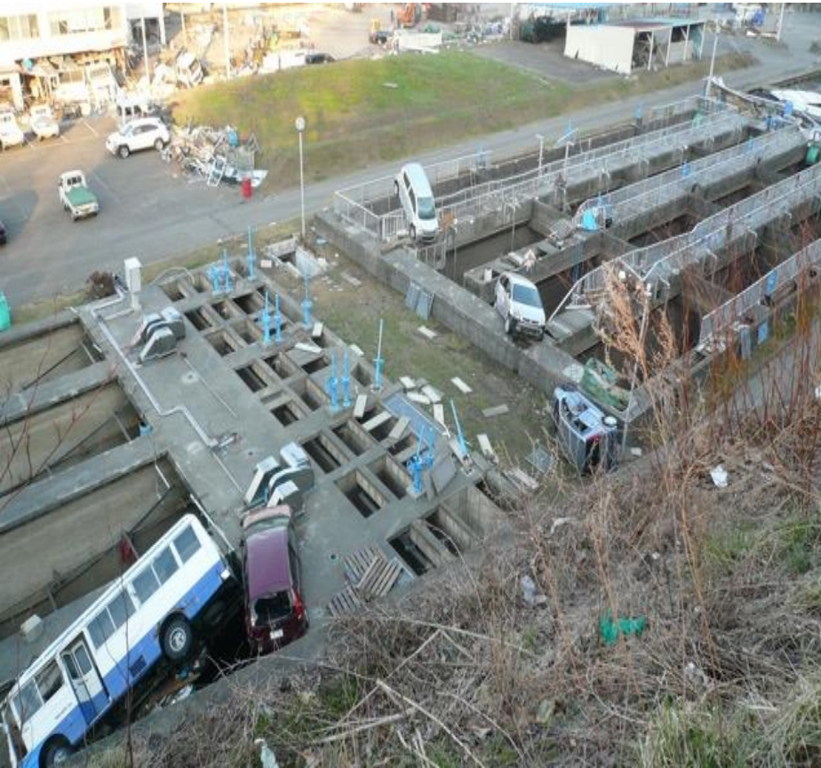
Destroyed sewage plant
