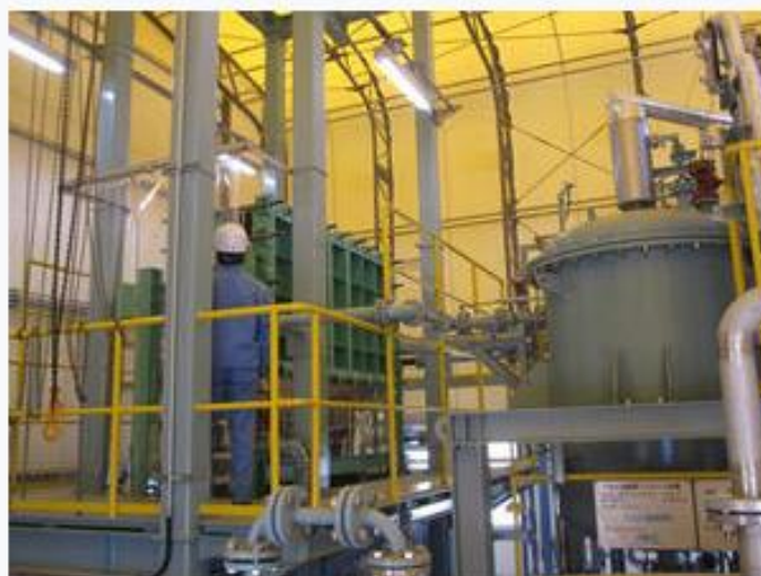
The large-scale alkaline water electrolysis plant
